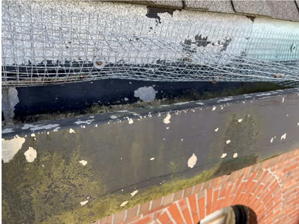
Photo 9: Close up of gutter with failing paint finish and deformed and detached leaf screen
