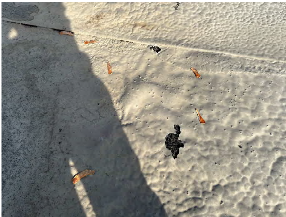
Photo 15: Close up of deteriorated roofing membrane that had a coating applied overtop
