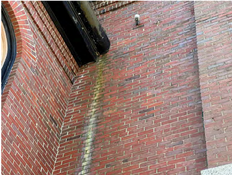
Photo 29: Overview of run-off and organics staining below gutter likely from overflow
