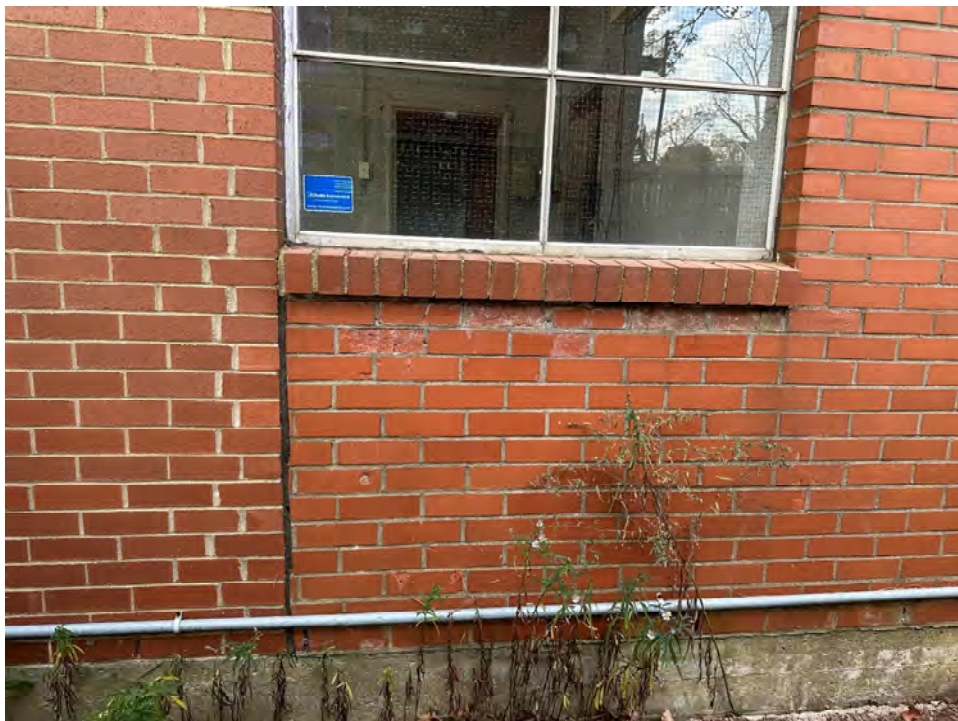
Photo 4: Brick deterioration on east elevation below brick sills
