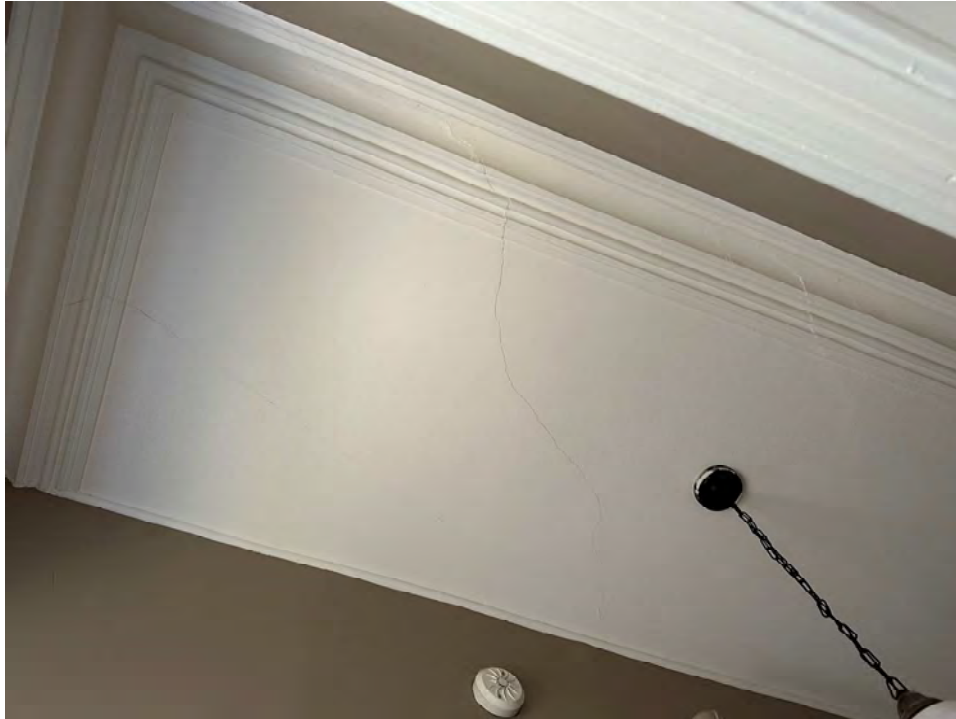
Photo 47: Cracking on ceiling inside building (typ. at several locations)
