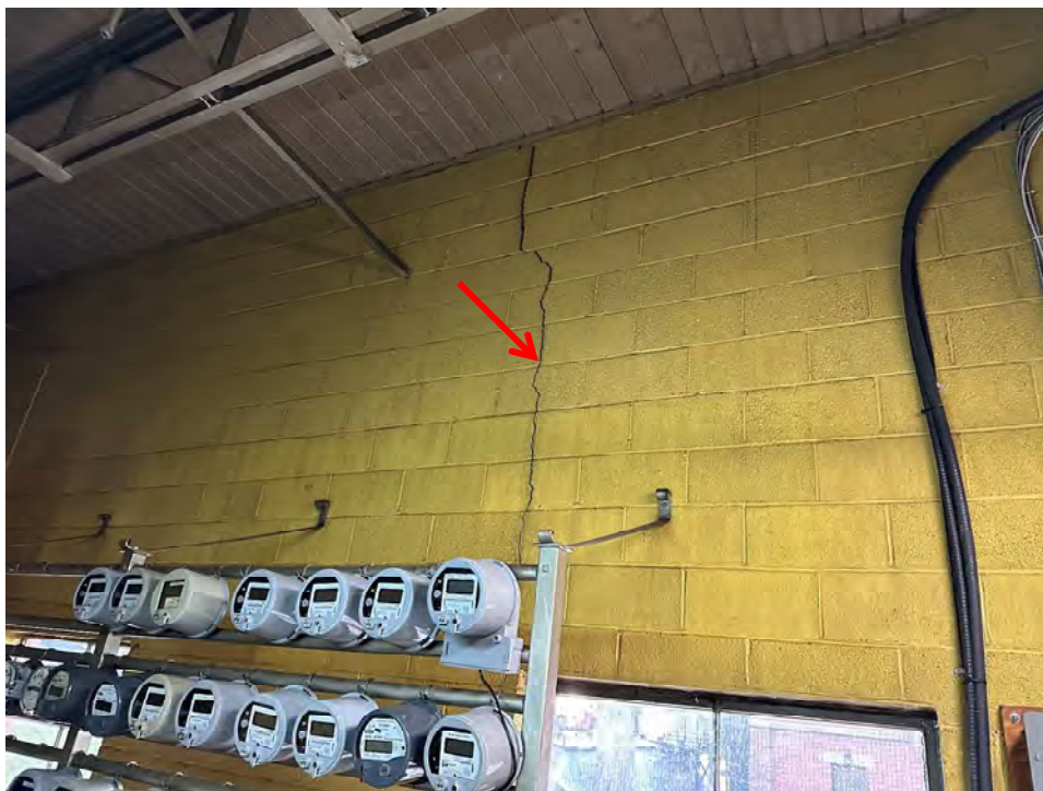
Photo 12: Full wall height CMU cracking adjacent to window opening on east elevation
