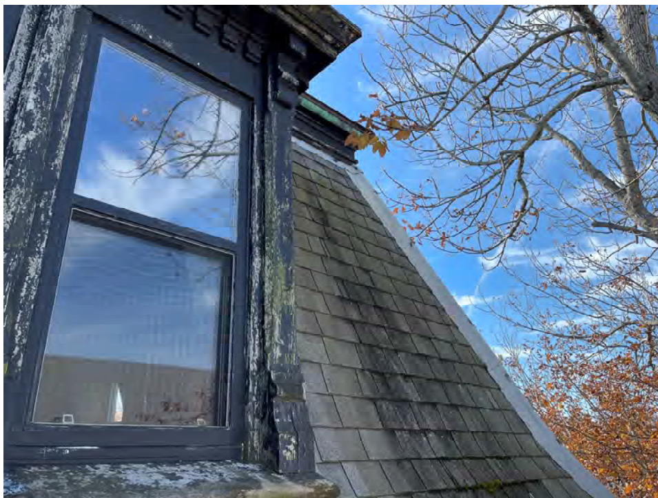
Photo 8: Stained asphalt shingle roofing around dormer window on steeply sloped Mansard roof face and failing window framing paint finish (north elevation)
