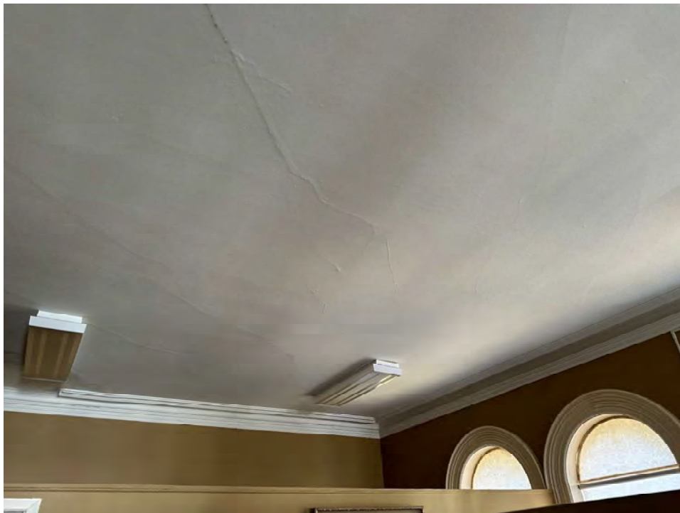
Photo 46: Cracking on ceiling inside building (typ. at several locations)
