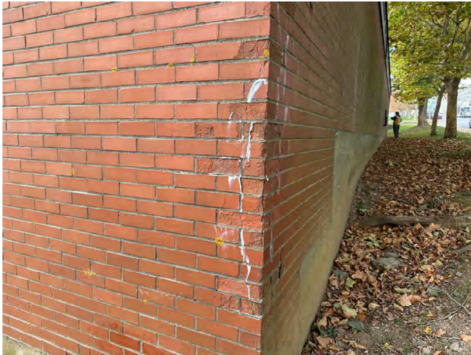
Photo 5: Brick deterioration at northeast corner
