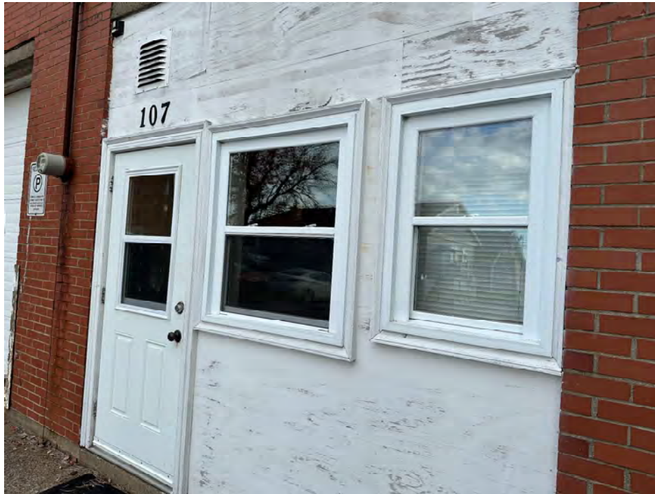
Photo 15: Newer door and windows at Electric Shop entrance set in older painted plywood cladding
