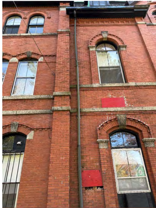
Photo 25: Overview of mortar joint deterioration in vicinity of west elevation downspout
