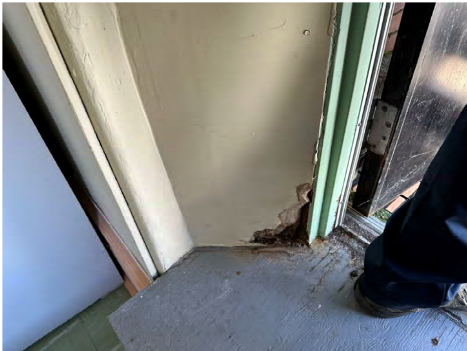
Photo 42: Moisture ingress deterioration at third storey fire escape door
