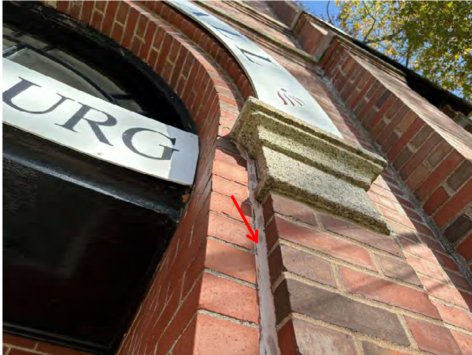
Photo 21: Sealant between different vintages of brick with cohesive tears
