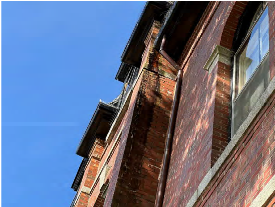
Photo 27: Overview of staining from gutter run-off on south elevation Cumberland Street entrance
