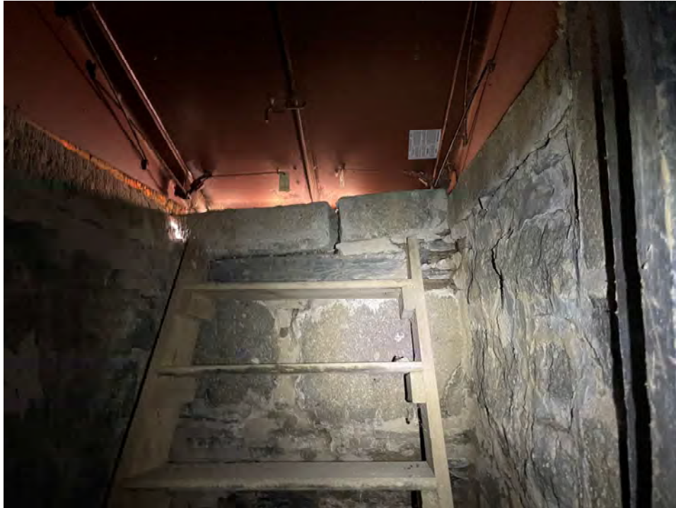
Photo 45: View from inside basement bulkhead hatch with daylight indicating no air or water seal in areas
