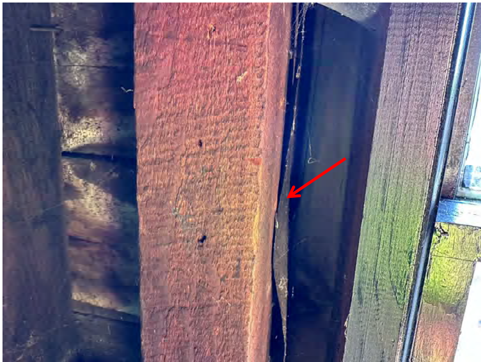
Photo 14: Building paper terminating inside attic/storage space at window opening
