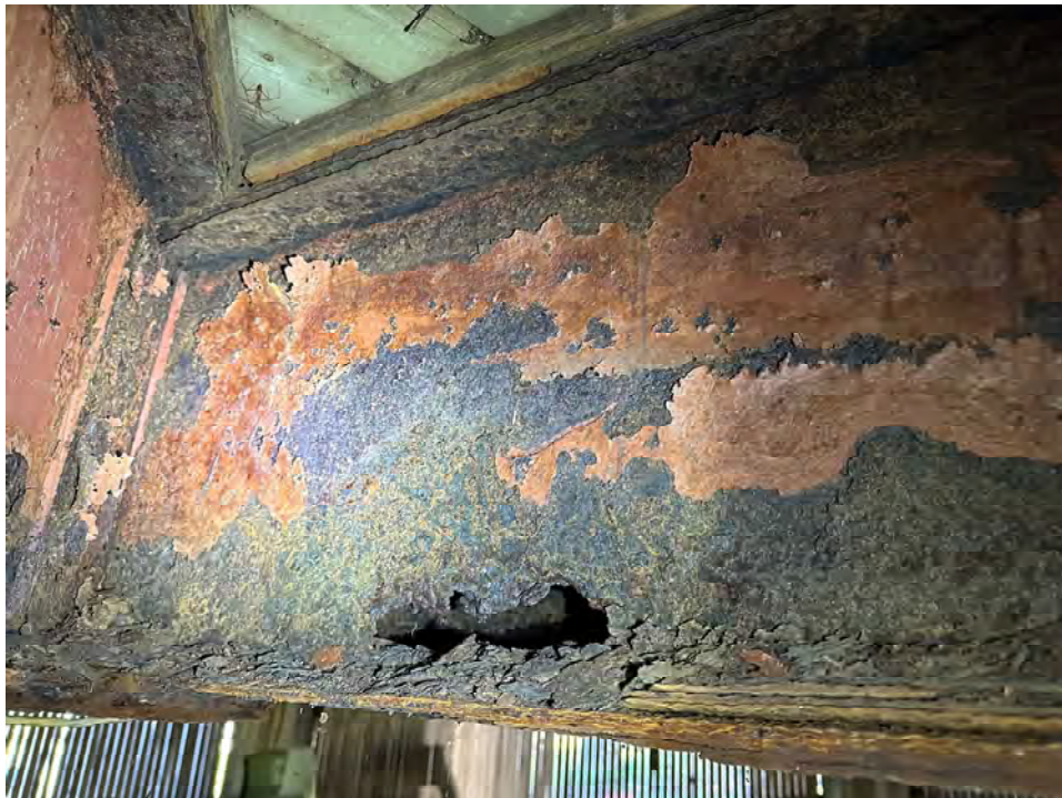
Photo 4: Full cross-sectional corrosion steel beam web
