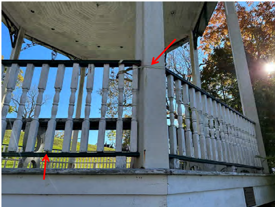
Photo 10: Guardrail with temporary strapping and loose balusters
