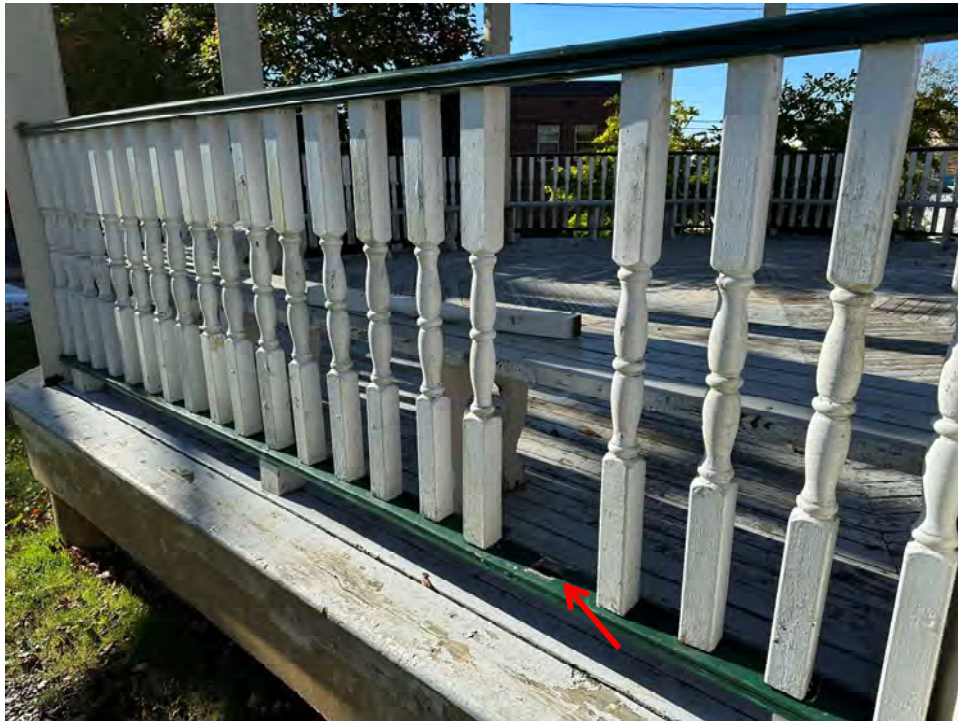
Photo 11: Section of guardrail with missing baluster
