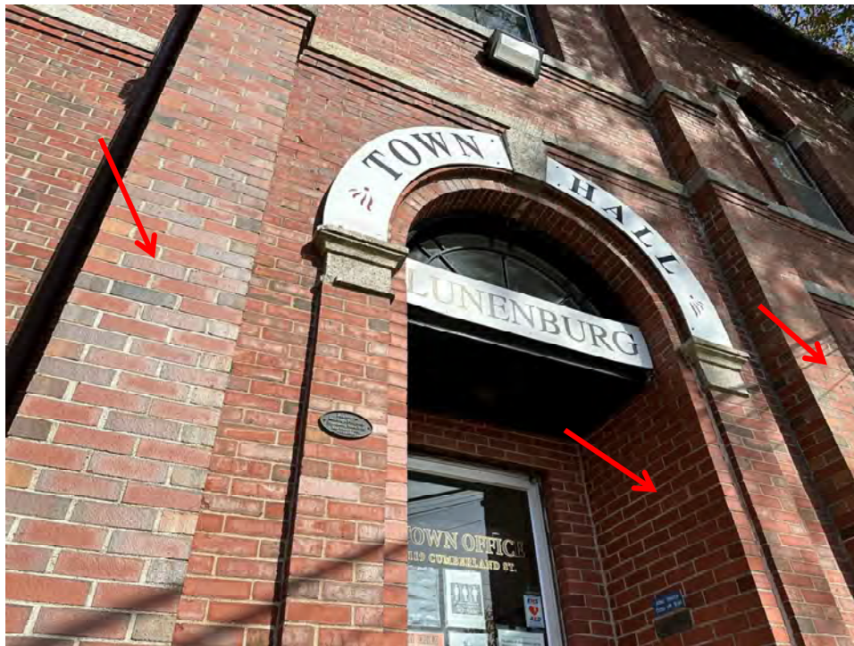
Photo 19: Existing brick repair areas near south elevation Cumberland Street entrance
