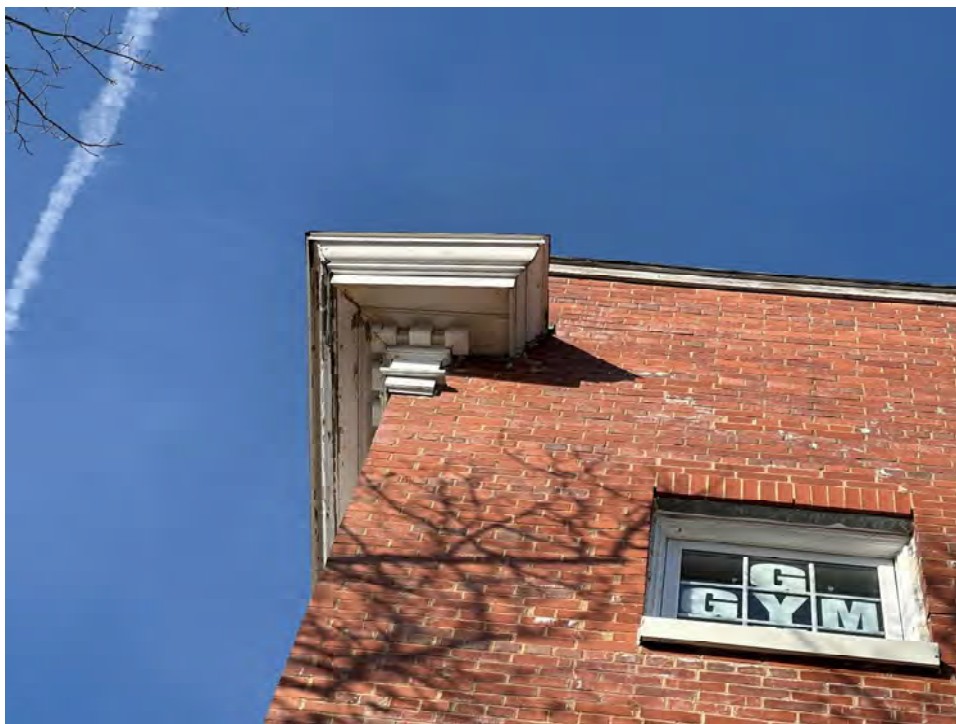
Photo 17: Failing paint finish and deterioration on underside of wood cornice at southeast corner
