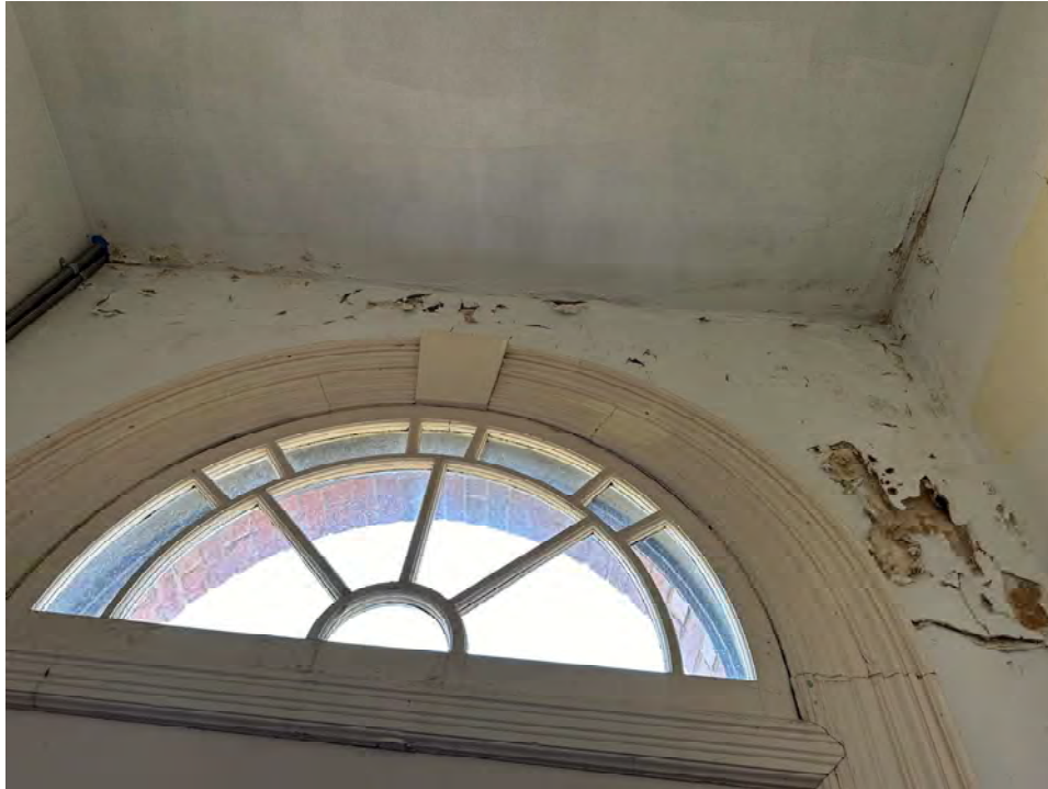
Photo 41: Moisture ingress deterioration above east elevation entrance
