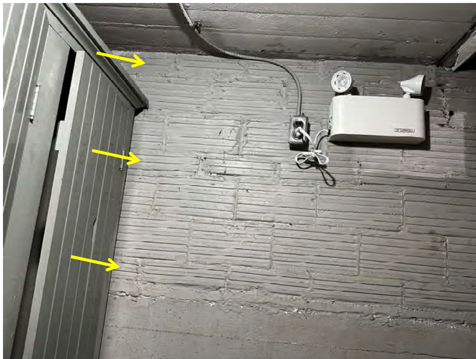
Photo 7: Structural clay tile as visible from building basement. Yellow arrows at on bed courses
