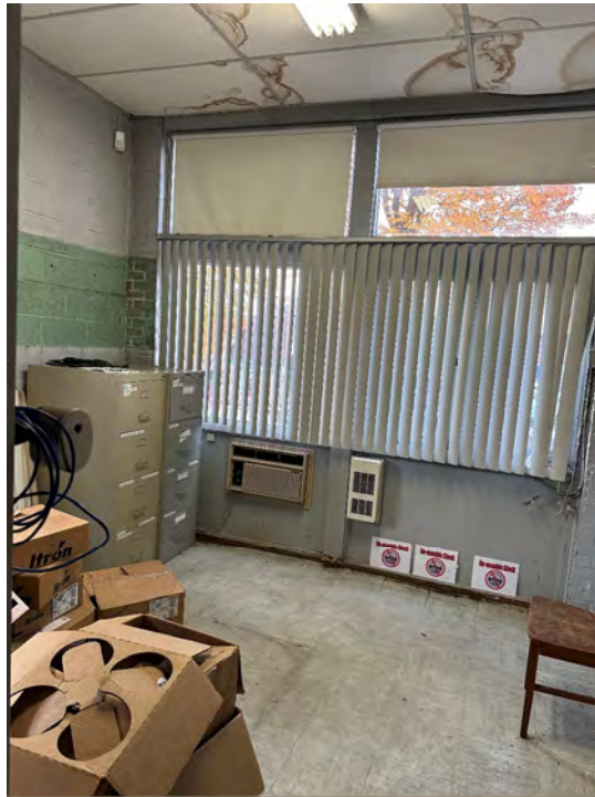
Photo 17: Deteriorated window unit as visible from building interior. Note, leakage staining on ceiling tiles above
