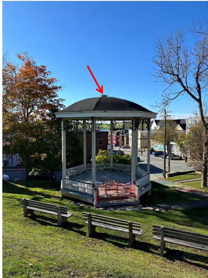
Photo 17: Ornament missing from roof of Bandstand
