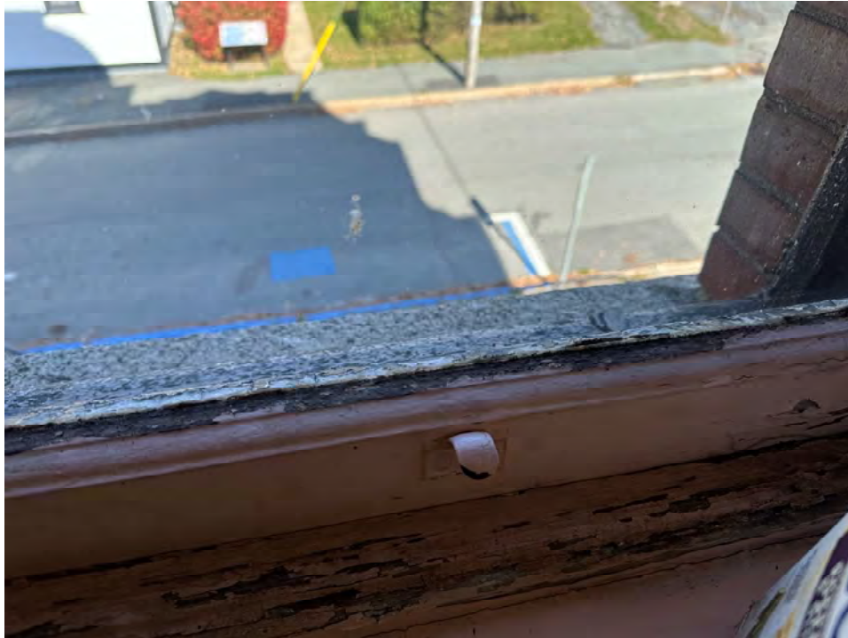
Photo 35: Peeling paint and deterioration on wood window, likely from condensation
