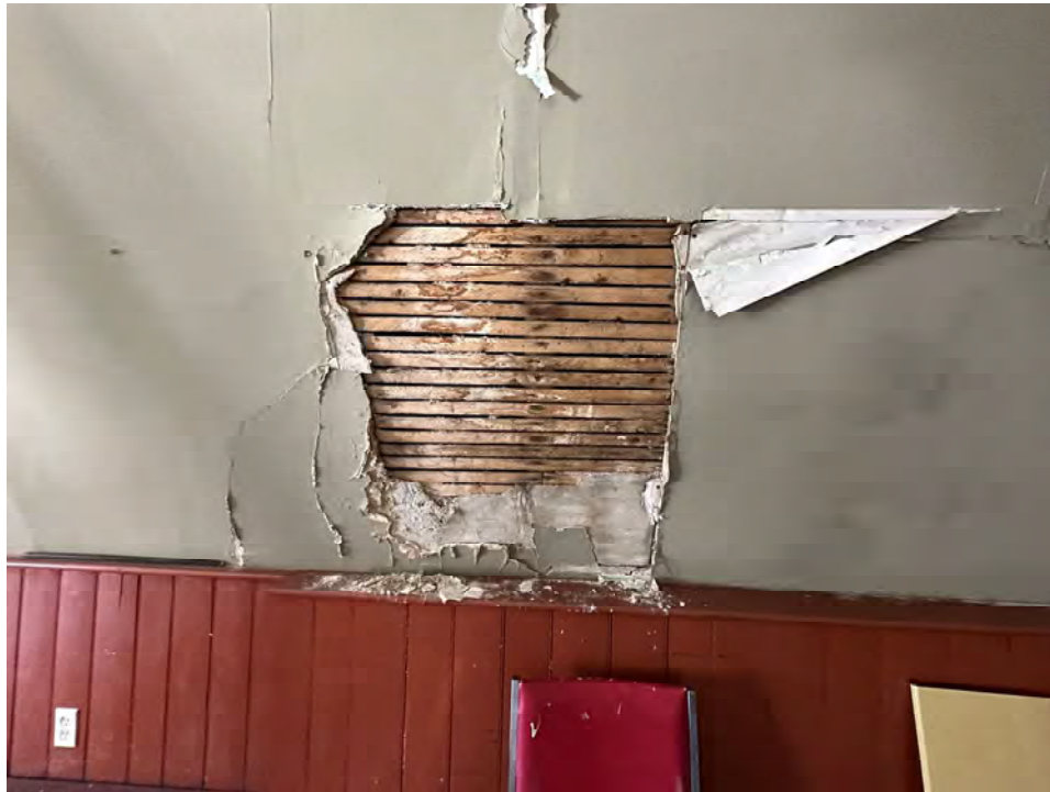
Photo 49: Deterioration from moisture ingress on third floor unoccupied space
