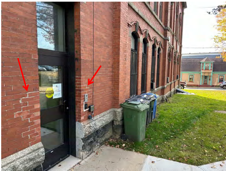
Photo 18: Existing brick repair areas near west elevation entrance
