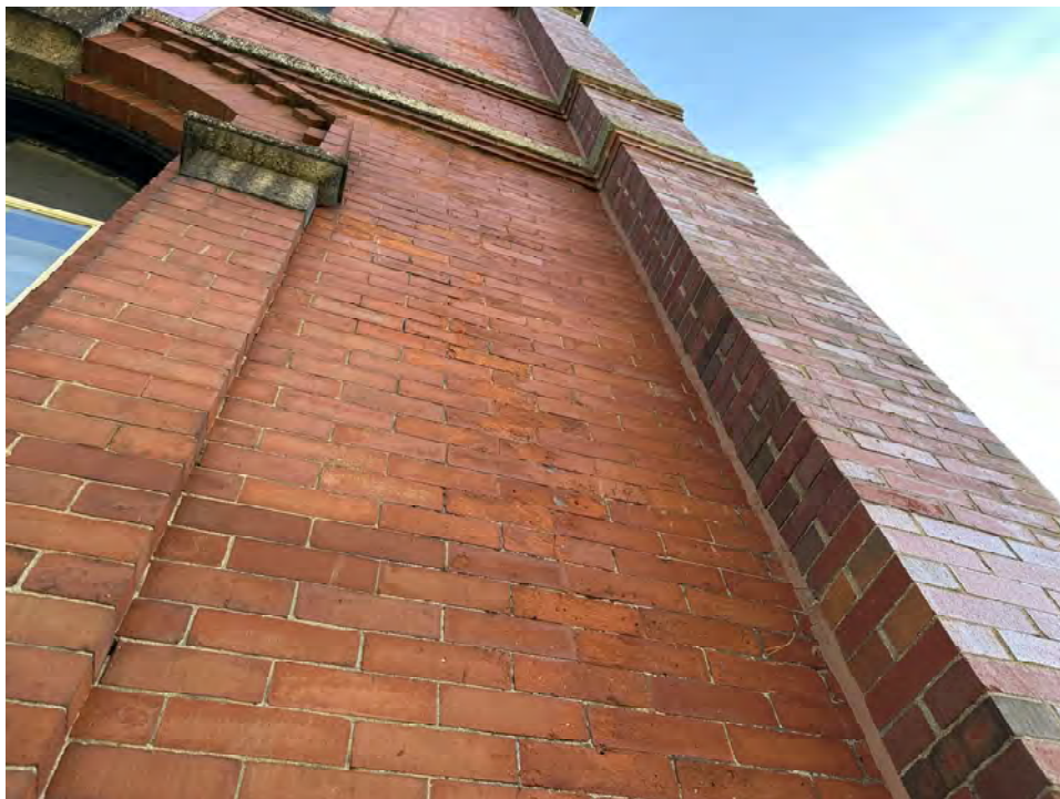
Photo 26: Overview of brick face spalling near southwest corner pilaster on west elevation
