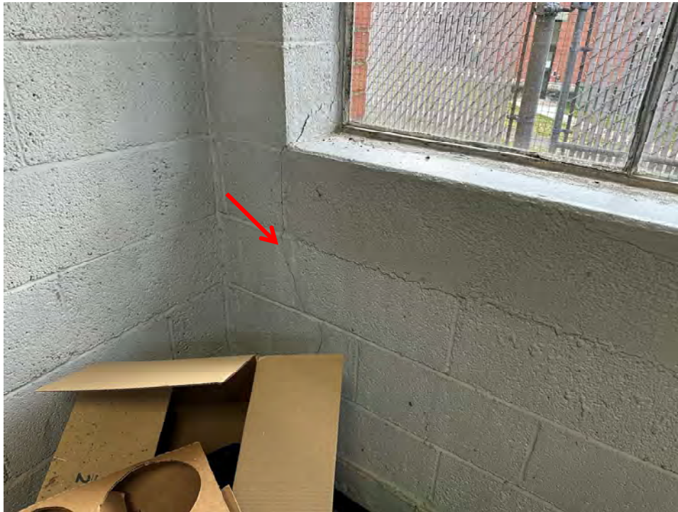
Photo 11: CMU cracking below window opening on east elevation wall
