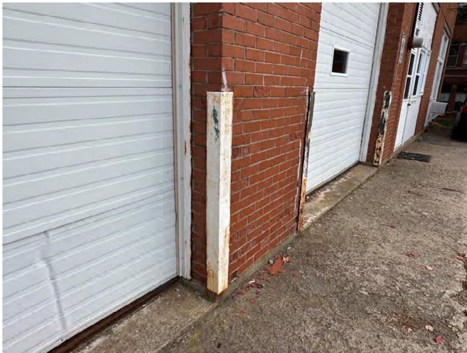
Photo 8: Brick deterioration on south elevation solid brick pier
