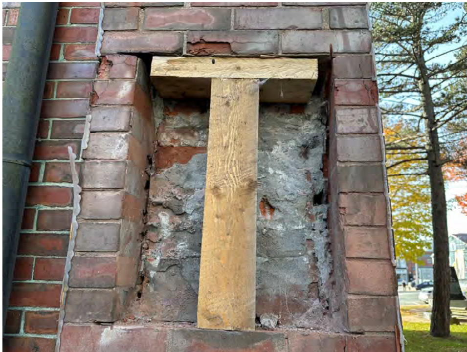
Photo 32: Exploratory opening on north face of northwest corner pilaster by others and reopened for RJC review
