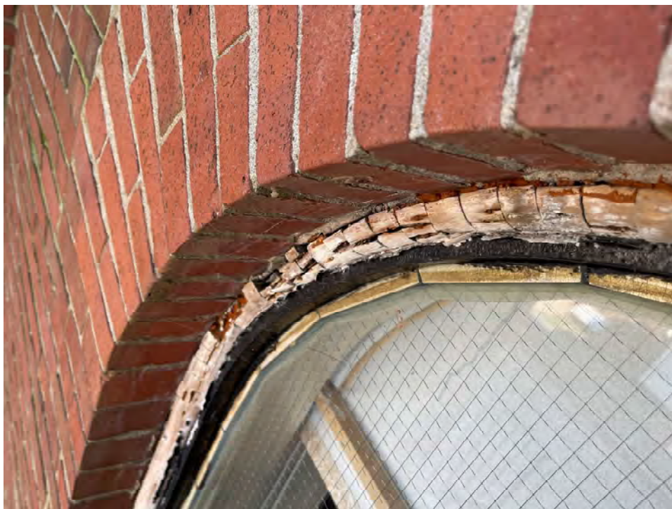
Photo 36: Peeling paint and deterioration of exterior wood detailing above retrofit vinyl window
