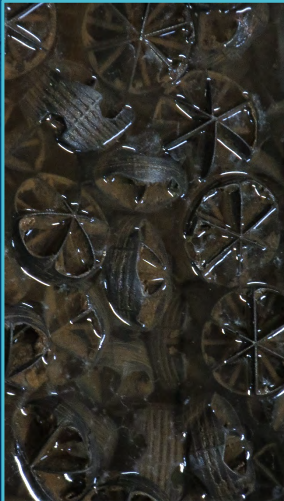
Bioreactor Tank Aeration
