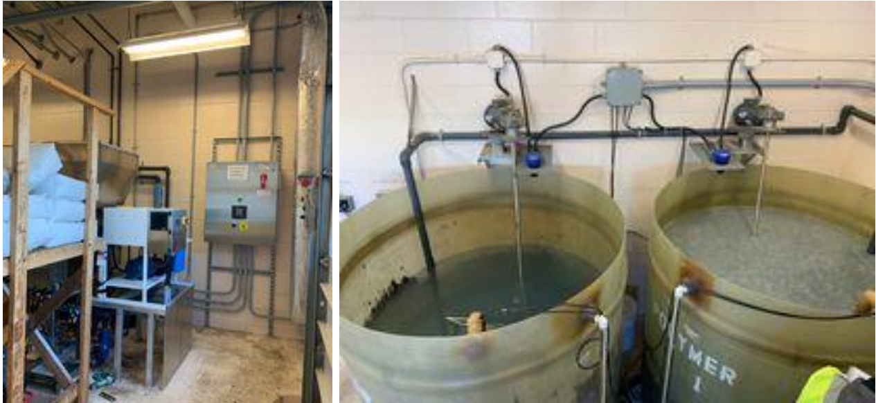
Figure 7 and 8: Existing Polymer Make-down System and Storage Tanks
