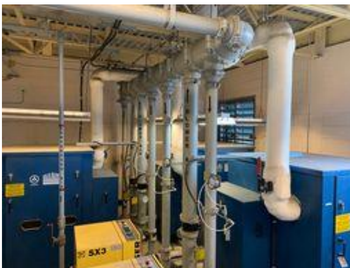
Figure 6: Existing Blower Room
