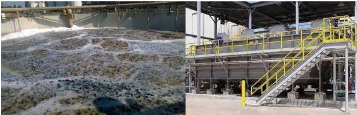
Figure 4 & 5: MBBR media and DAF unit
