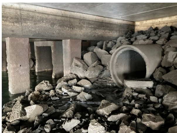
Figure 1.1: Existing effluent outfall (round pipe at right). Photo taken approximately 1 hour before low tide (2021-03-11 12:35).
