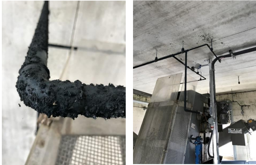
Figure 2 and 3: Existing Water Piping Headworks
