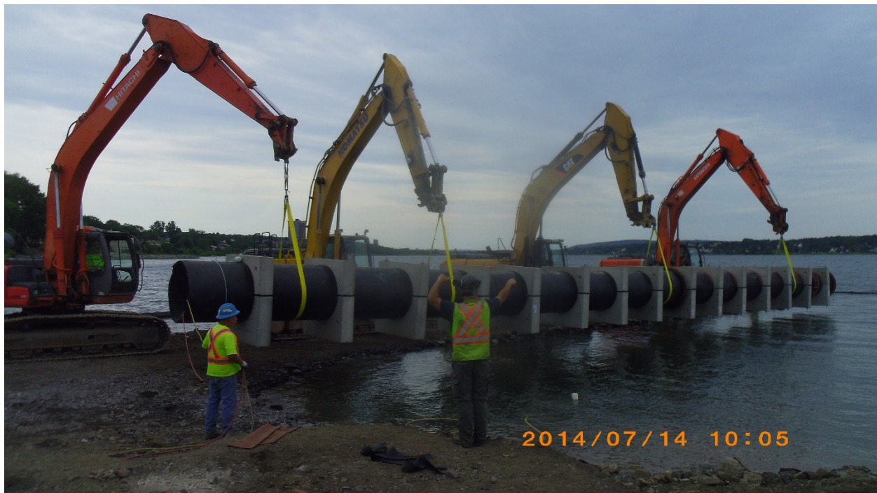
Figure 3.2: Installation of sewer outfall in Sydney Harbour. Pipe is HDPE and has concrete collar weights for ballast similar to what is proposed for the TOL outfall
