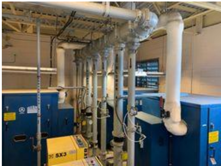
Figure 6: Existing Blower Room
