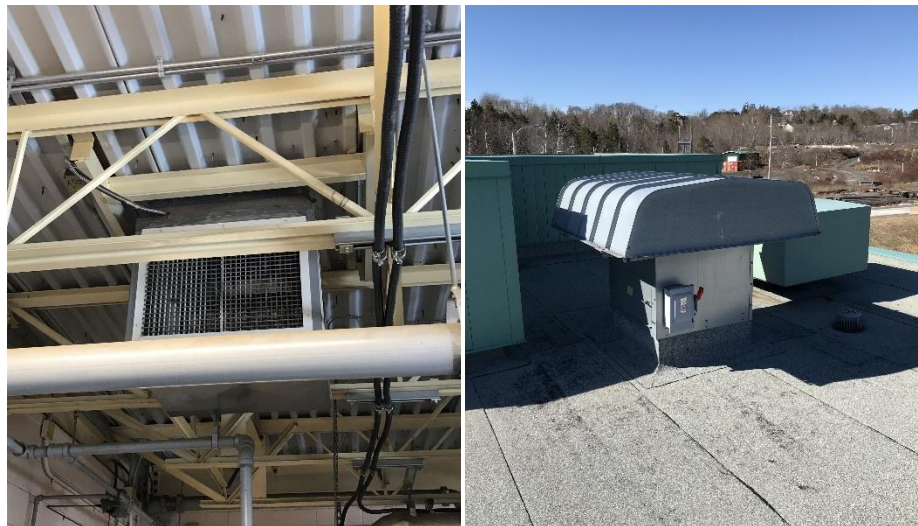
Figure 9 and 10: Existing HVAC equipment to service the blower room
