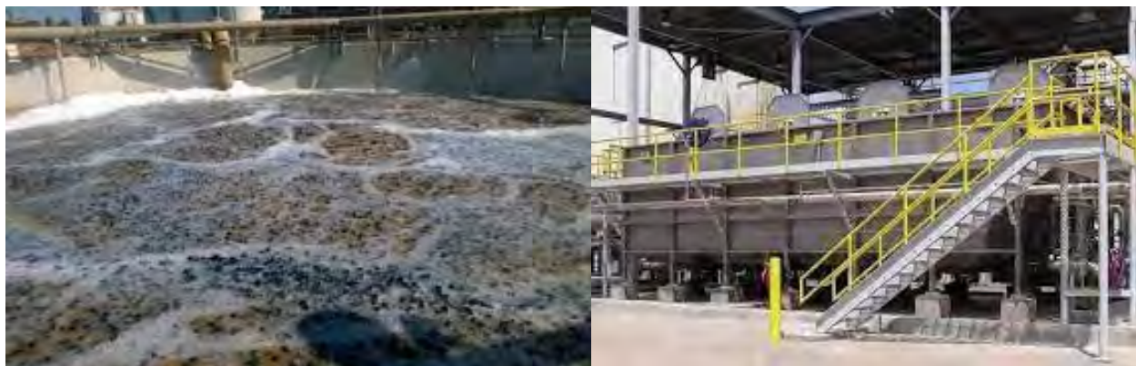
Figure 4 & 5: MBBR media and DAF unit
