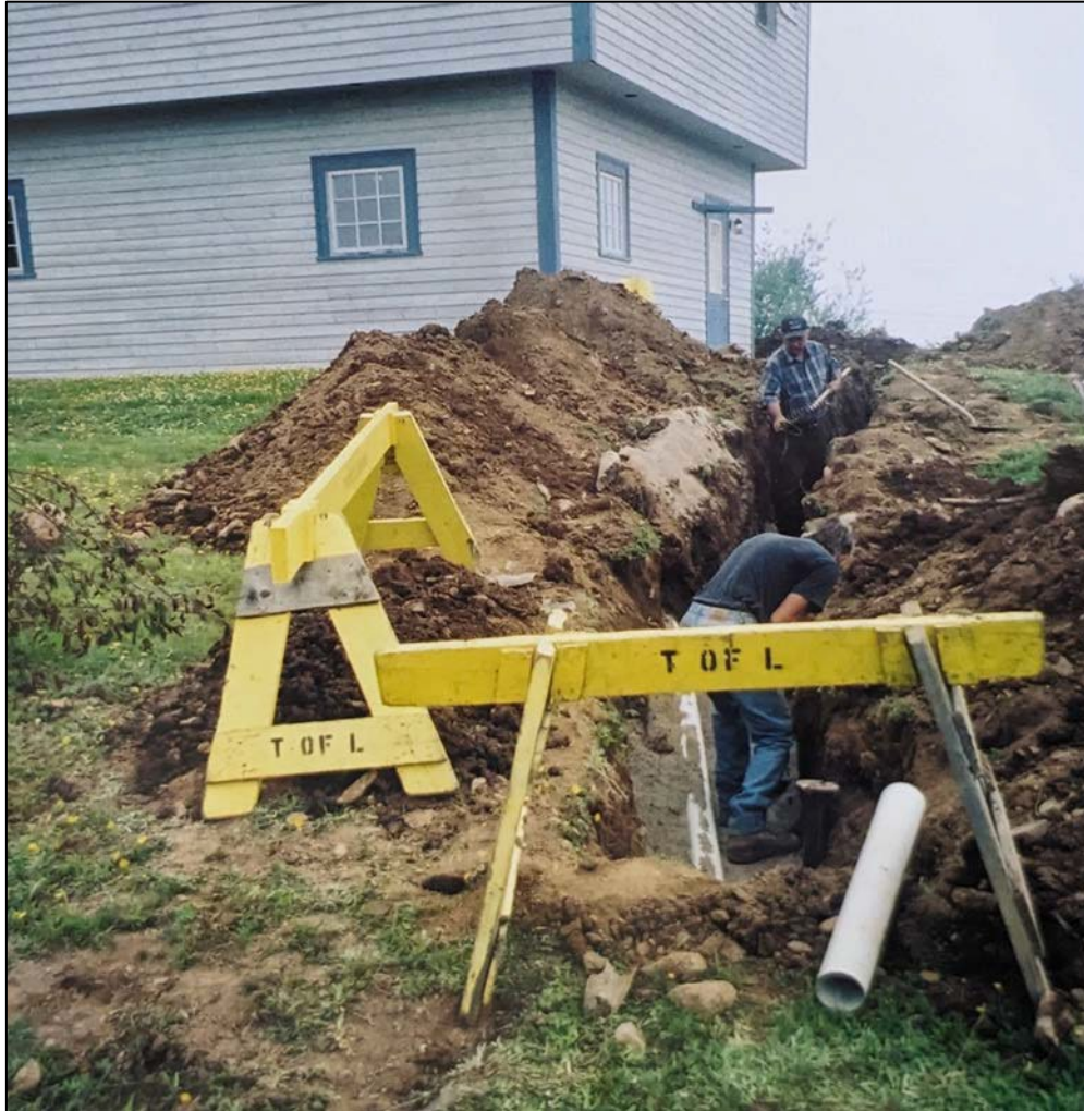
Figure 4-25: Sewer improvements in November/December 1999 on the southeast side of the VIC, looking northeast. Courtesy of Lunenburg Board of Trade.
