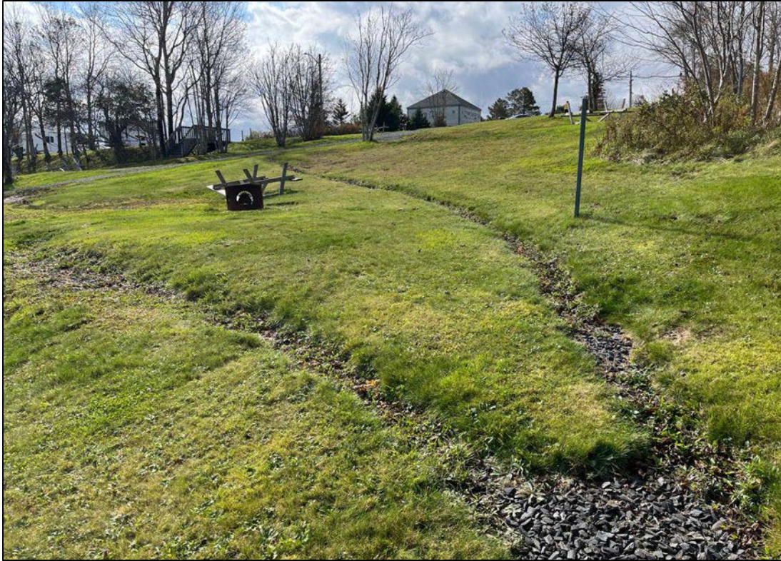
Plate 9: Gravel drains in the slope of the lower campground, facing south.
