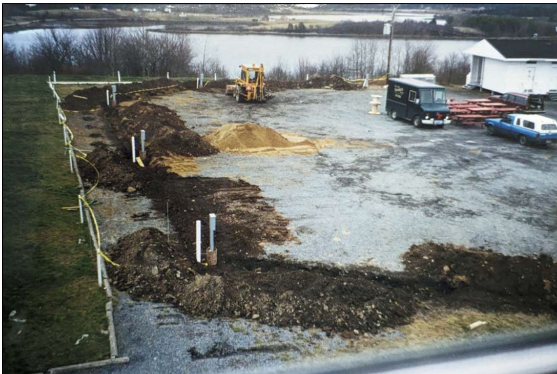
Figure 4-24: Electrical upgrades in November/December 1999 showing showers at top right and the Back Harbour in background, looking north.
