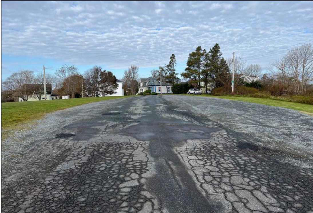
Plate 2: Blockhouse Hill Road, an asphalt road with wide gravel shoulders which separates Sylvia Park from the study area (located to the right), facing northwest towards the intersection of York Street and Kempt Street.
