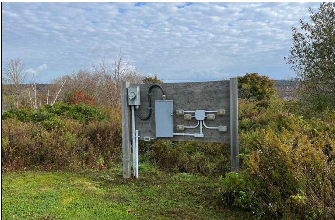
Plate 3: An electric meter along the edge of the study area and Blockhouse Hill Road, indicating the presence of buried utilities, facing northeast.
