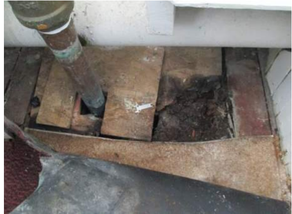
Figure 92 – Hole in floor at base of knee-wall – wet wood is soft.
