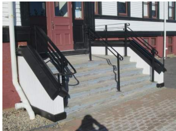
Figure 9 – RHS (right-hand side) Entry stair rebuilt in 2016, Guardrails installed in 2018 – good condition. Failed paint on steps and landing.
