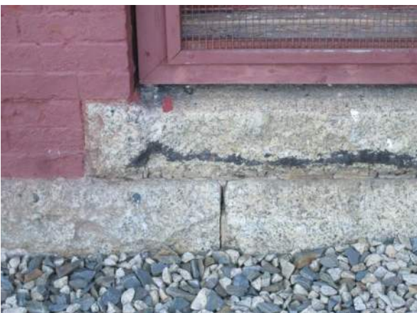
Figure 28 – Open joint in stone band below stone sill on far LHS basement window.
