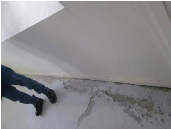
Figure 99 – Rotted door trim and baseboard above damp section of floor.
