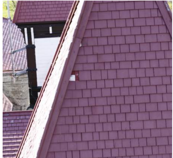
Figure 58 – Tower 2. North Elevation. Area with the missing shingles, which can be a possible cause of rainwater penetration.
