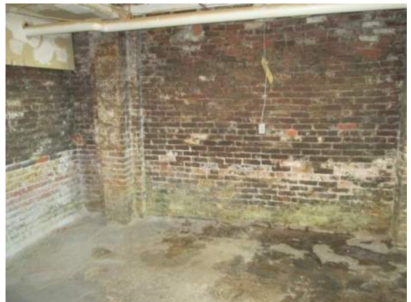
Figure 82 – Interior brick wall in room B24. Rising damp at bottom and efflorescence.
