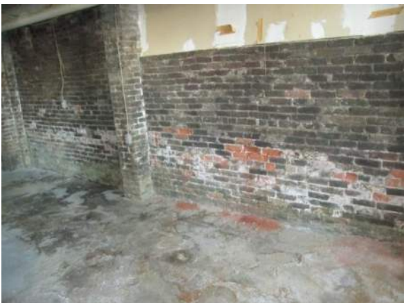
Figure 83 – Interior brick wall in room B24, rising damp at base bricks and deteriorating/crumbling brick above.
