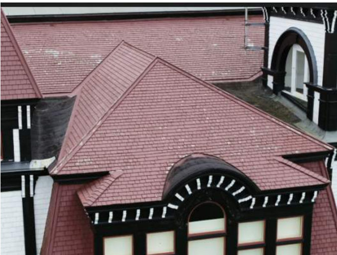
Figure 73 – West Elevation (Center). Some areas of peeled and faded Red Stain
