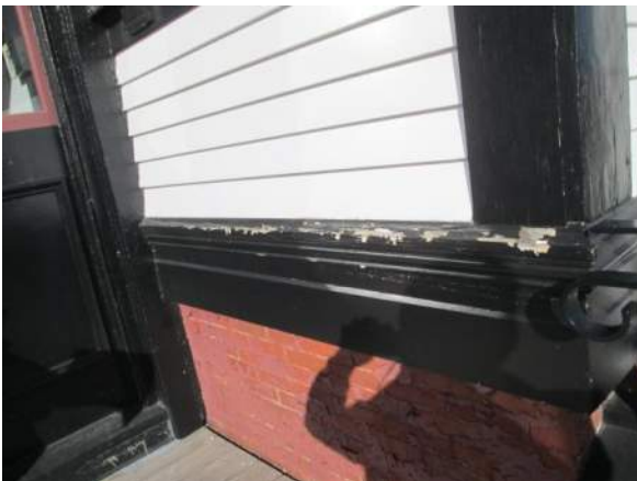
Figure 8 – Peeled paint on top of wood sill above brick foundation at LHS entry doors. This work completed in 2020.
