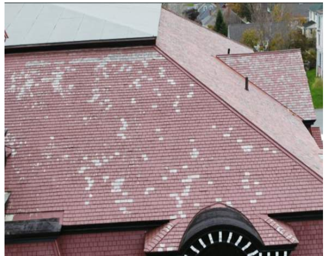
Figure 74 – West Elevation (Right side). Significant areas of peeled and faded Red Stain
