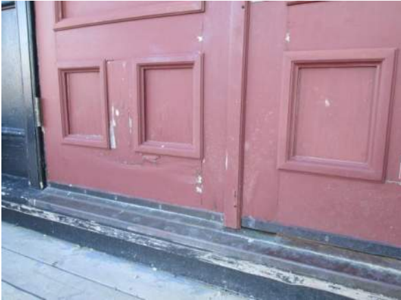
Figure 30 – Doors refinished in 2018. Gaps at threshold and between doors. Paint failure on doors and wood sill.
