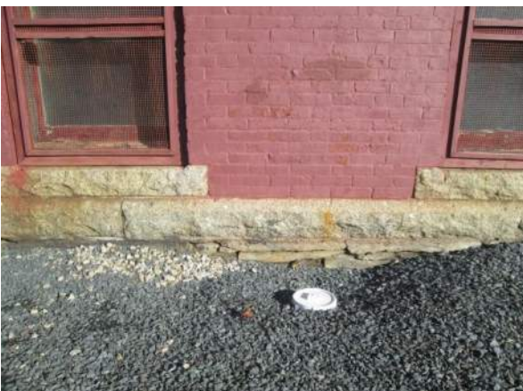
Figure 37 – Open joint in stone band below stone sill and large open joints in exposed foundation stones below band. Typical paint conditions on brick foundation wall.
