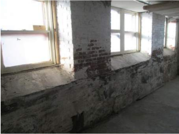
Figure 75 – Paint failure in brick section of foundation wall. Paint failure on lower stone section of wall also locations of efflorescence.
