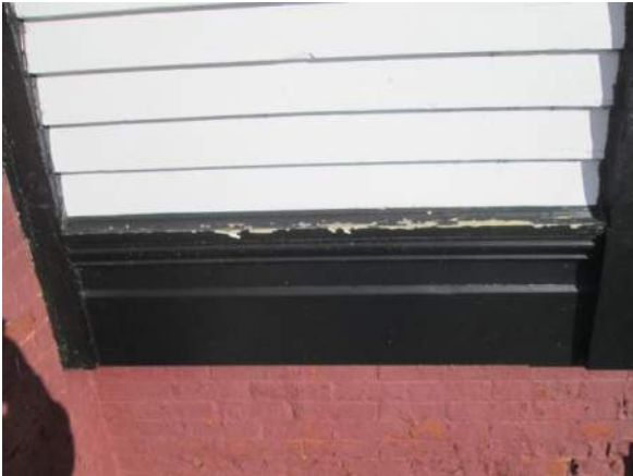
Figure 4 – Peeled paint on top of wood sill at LHS entry return.
