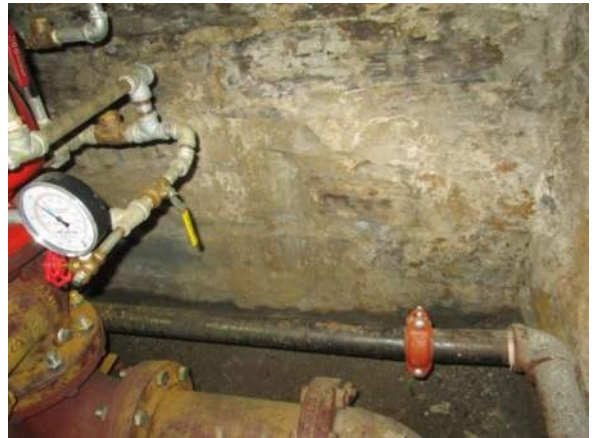
Figure 94 – Room B25: damp section on floor against foundation wall.
