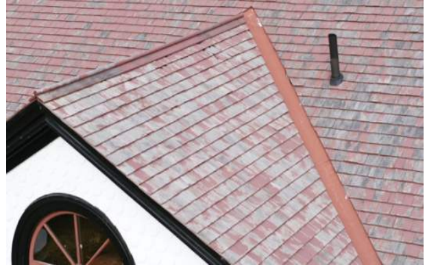
Figure 64 – South Elevation (center). A significant areas of peeled and faded Red Stain
