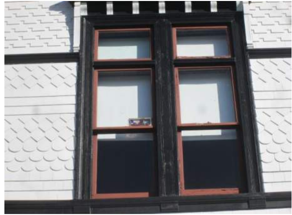
Figure 46 – Paint failure on transom, upper and lower sash on right hand side.
