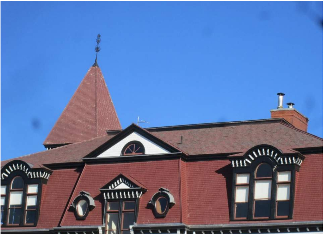
Figure 47 – South Elevation: Mansard Roof. Upper section of mansard roof replaced in 2018. Appears that stain is failing. Tower roof beyond also exhibits signs of faded and worn finish stain.
