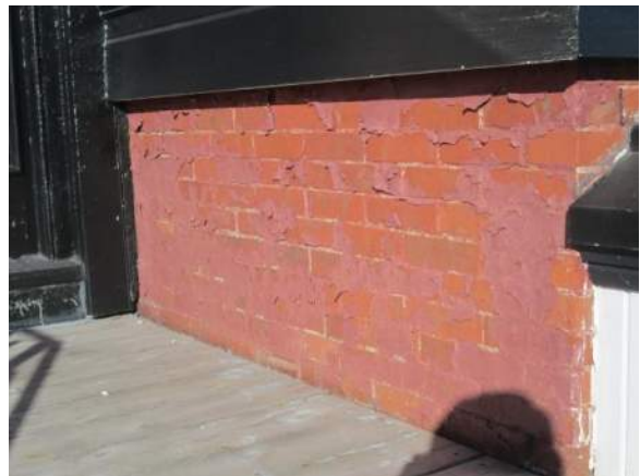
Figure 7 – Complete paint failure on brick foundation top of landing.
