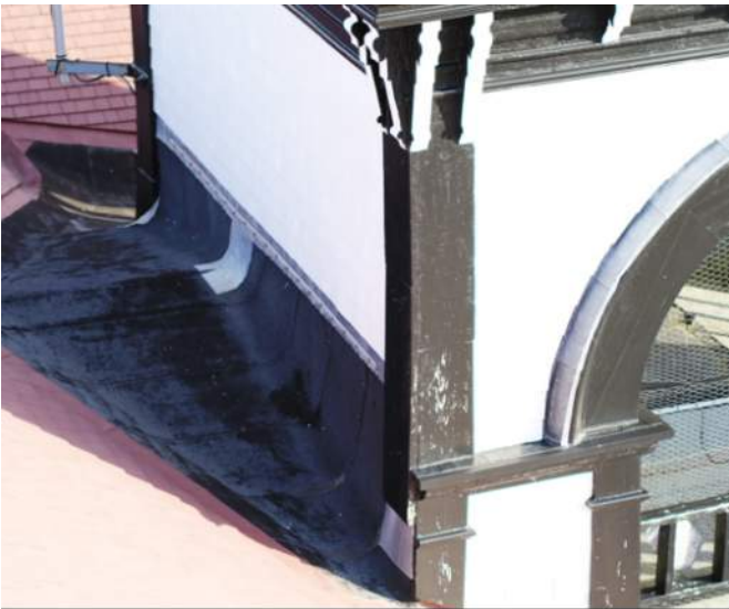
Figure 53 – Tower 3. South Elevation. Paint flaking at some areas
