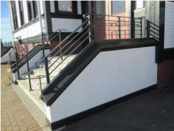
Figure 10 – RHS entry stair rebuilt in 2016 – good condition. Guardrails in 2018 – good condition.
