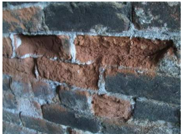
Figure 84 – Deteriorating / crumbling brick.
