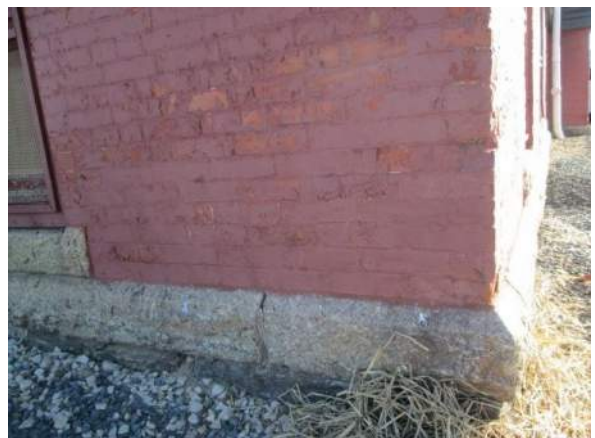
Figure 35 – Small open joint in stone band. Spalled brick and typical paint failure on brick foundation: South-West corner.
