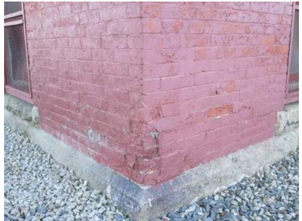
Figure 21 – North-West corner brick foundation: brick is broken, spalled and cracked. Typical paint conditions.
