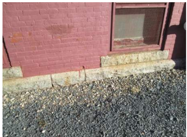
Figure 38 – Spalled brick and typical paint failures. Open joint in stone band below brick.
