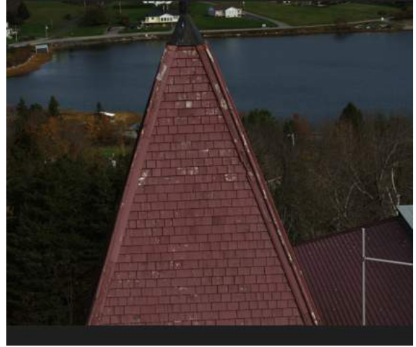
Figure 60 – Tower 1. South elevation. A significant areas of peeled and faded Red Stain
