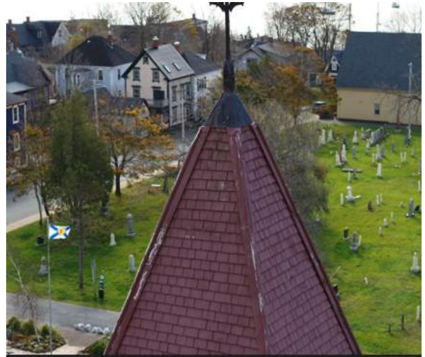
Figure 62 – Tower 1. North Elevation. Shingles at the top areas of the Tower roof are covered with mold. Some areas of peeled and faded Red Stain
