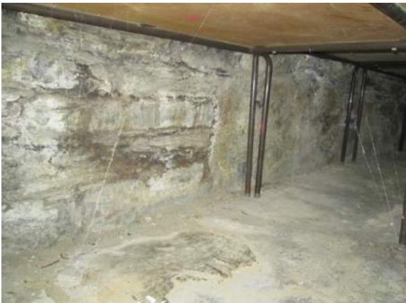
Figure 79 – Stone foundation wall below windows show some locations of efflorescence.
