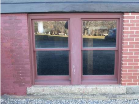
Figure 32 – New windows installed in 2018 – faded paint.
