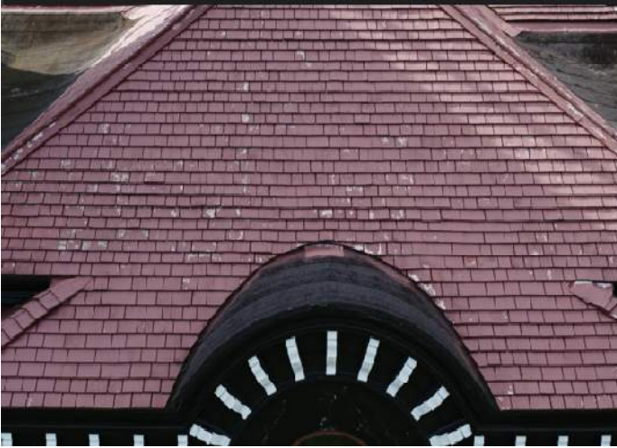
Figure 59 – West elevation. Areas with peeled and faded Red Stain
