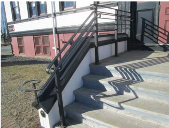
Figure 6 – Entry stair rebuilt in 2017, Guardrails installed in 2018 – good condition. Failed paint on steps and landing.
