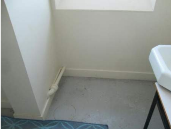
Figure 87 – Inside former washroom space: room is dry with no damp / wet locations noted.
