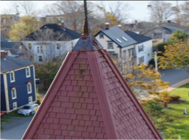
Figure 55 – Tower 3. North Elevation. Shingles at the top areas of the Tower roof are covered with mold
