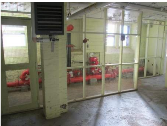
Figure 95 – Sprinkler pump against west wall.
