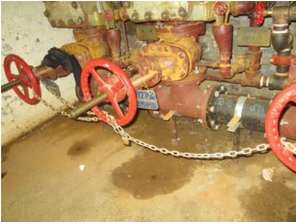
Figure 93 – Room B25: water on floor against foundation wall.
