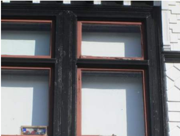
Figure 45 – Paint failure on upper transom sash.
