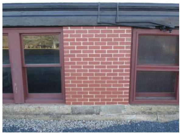
Figure 33 – New brick foundation wall section re-installed in 2018 when old access doors used to be.
