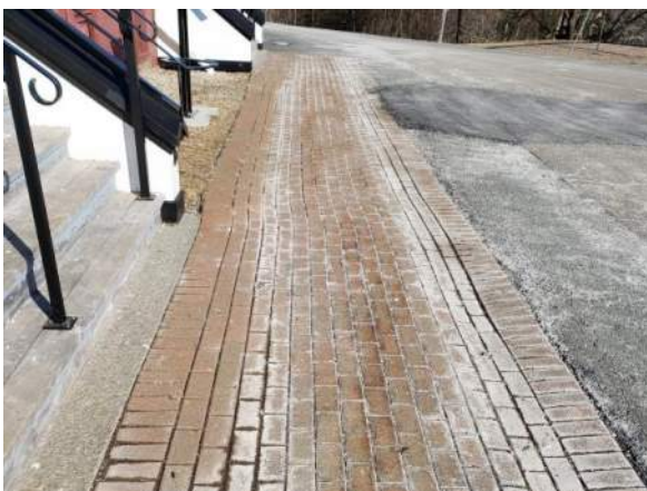
Figure 14 – Brick paver stone walkway. Sunken and “heaved” locations create an uneven walking surface, potential tripping hazard. Looking North.
