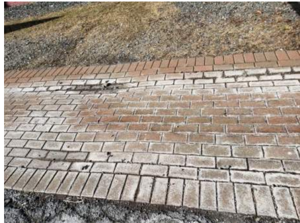
Figure 13 – Brick paver stone walkway. Sunken and “heaved” locations create an uneven walking surface, potential tripping hazard.
