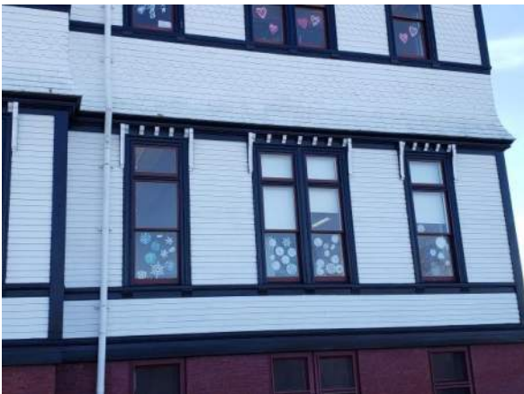
Figure 22 – Minor paint chipping and environmental staining on curved section of shingles above ground floor windows – typical across the North elevation.
