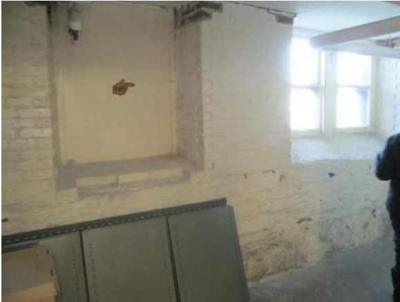
Figure 85 – Foundation wall outside former boys washroom: No wet or damp locations noted
