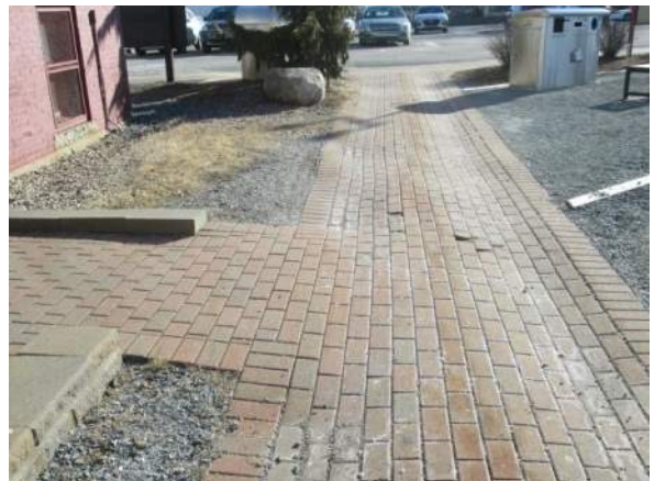
Figure 44 – Brick paver sidewalk from South “accessible” entrance: Heaving and sunken areas. Potential tripping hazard.
