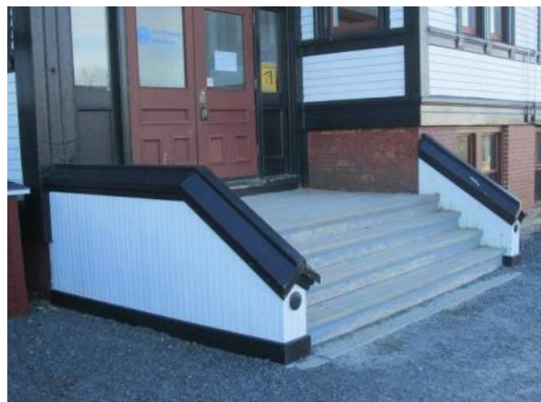
Figure 29 – Entry stair LHS rebuilt in 2016 – good condition. Paint on steps and landing is worn.
