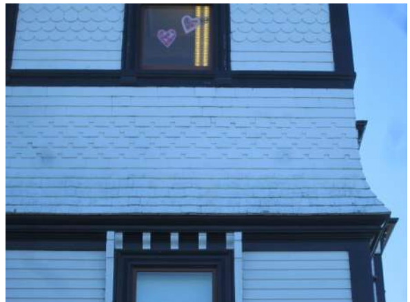
Figure 23 – Minor paint chips and environmental staining on curved section of shingles.
