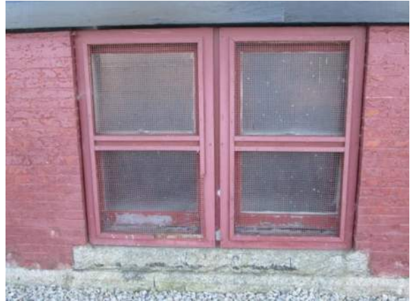
Figure 19 – Basement storm/security windows fairly poor condition. Typical at all locations on basement windows.
