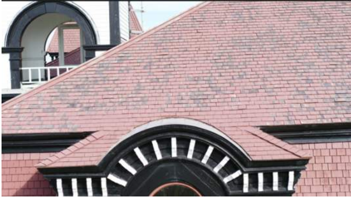
Figure 63 – South Elevation (left side). A significant areas of peeled and faded Red Stain
