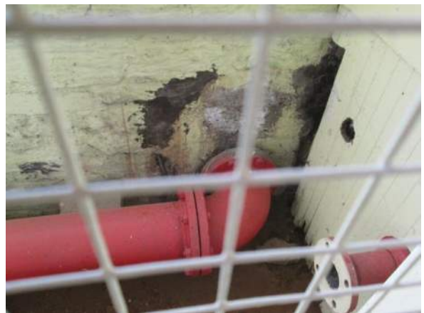
Figure 96 – Sprinkler pump line through stone foundation wall. Wall and floor appear to be damp.
