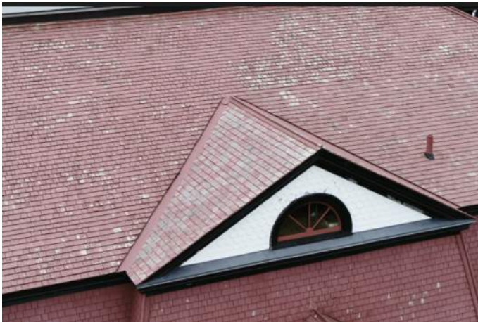
Figure 69 – North Elevation (Center-view1). A significant areas of peeled and faded Red Stain
