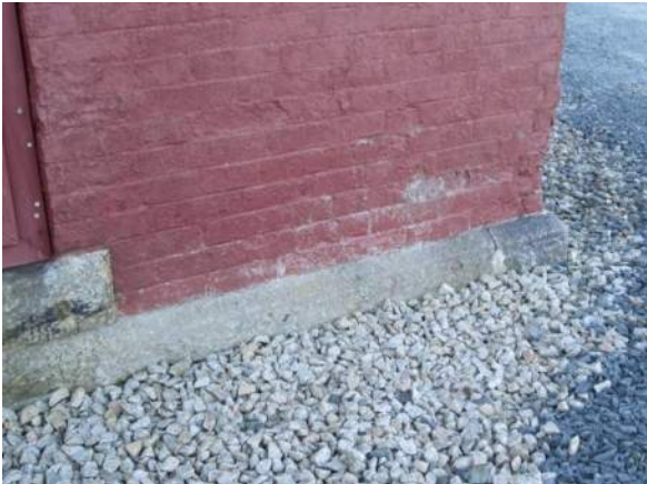
Figure 20 – Brick foundation, far RHS with spalled brick and failed paint finish – typical.
