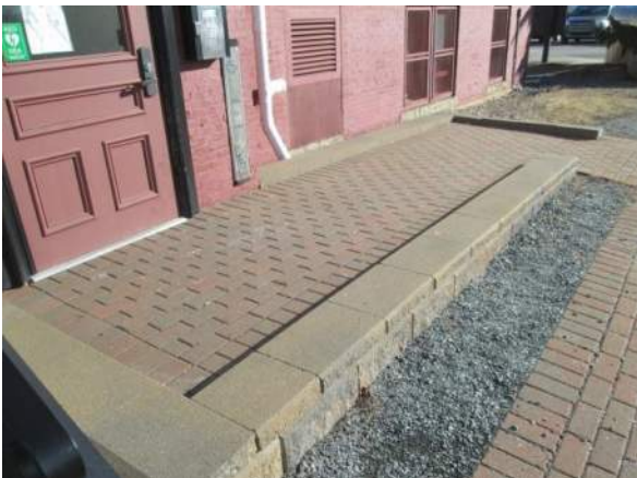
Figure 43 – Existing ramp to door – not code compliant.
