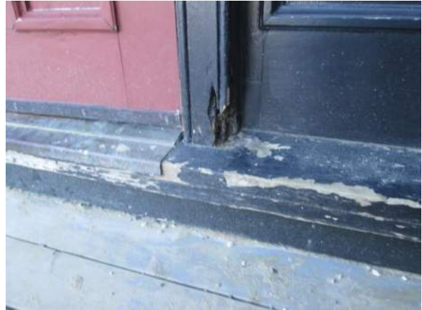
Figure 31 – Location of rot not repaired in 2018. Peeling paint on wood sill.
