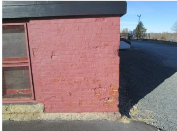
Figure 11 – Brick foundation at North-East corner, typical paint failure and heavy paint build up. Plug from staging support remains in brick and should be removed.
