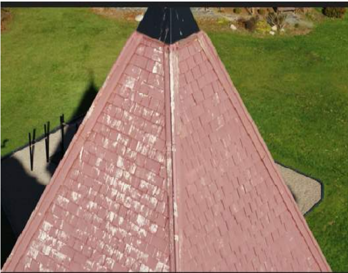
Figure 57 – Tower 2. South Elevation. A significant area of peeling and faded Red Stain
