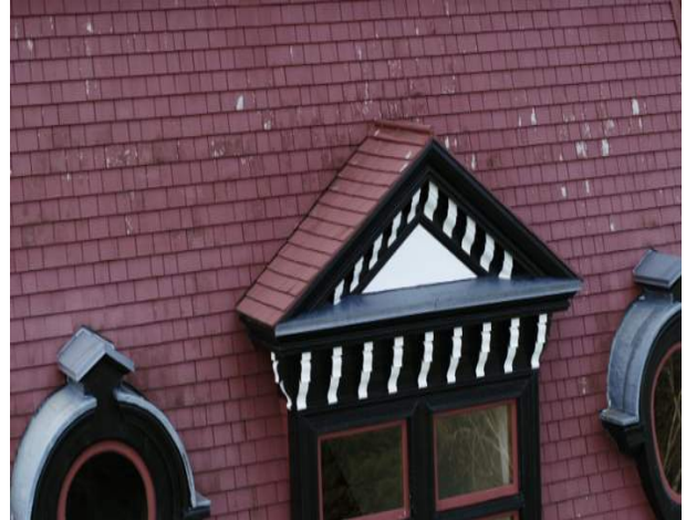
Figure 56 – South elevation. Areas with mold and peeled and faded Red Stain
