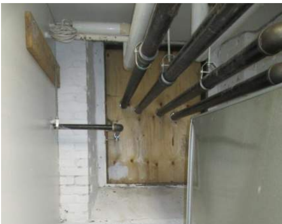
Figure 89 – Furnace oil line to the exterior (North elevation).
