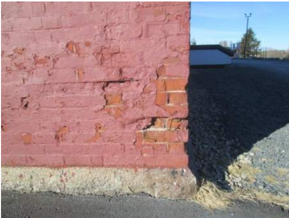
Figure 12 – North-East corner, broken & spalled brick. Typical heavy build up of paint and paint failure.
