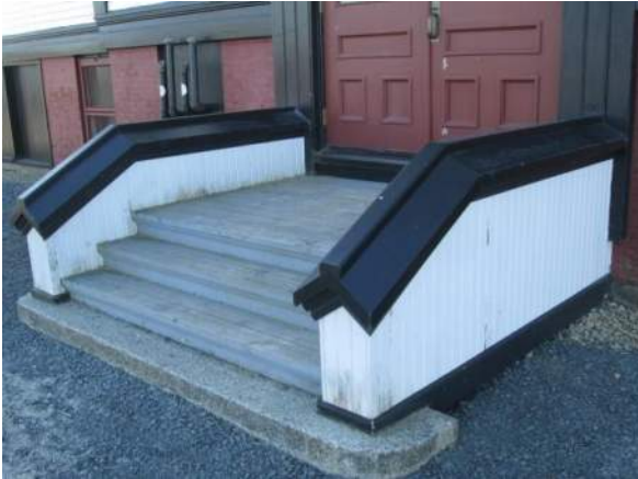
Figure 18 - Stairs to North doors rebuilt in 2016 - good condition. Steps and landing paint is worn off.
