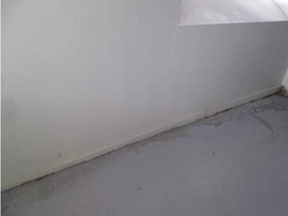
Figure 97 – Room at South-west corner of basement: floor is wet under baseboard.
