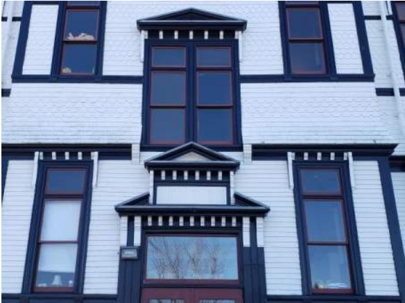
Figure 24 – Minor paint chips and environmental staining on curved section of shingles.
