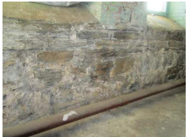
Figure 90 – Room B27 wall is dry and appears to be in good condition.
