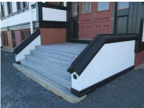
Figure 34 – Entry stair RHS rebuilt in 2016 – good condition. Paint on steps and landing is worn.
