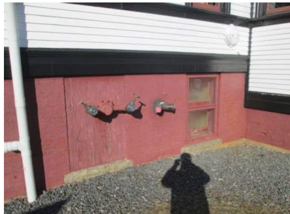
Figure 3 – Brick foundation wall with typical paint failures (peeled and cracked). Paint failure on plywood panel also.
