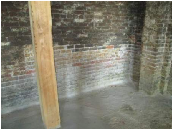
Figure 81 – Heavy efflorescence on interior wall of B24. New heavy timber post in foreground.
