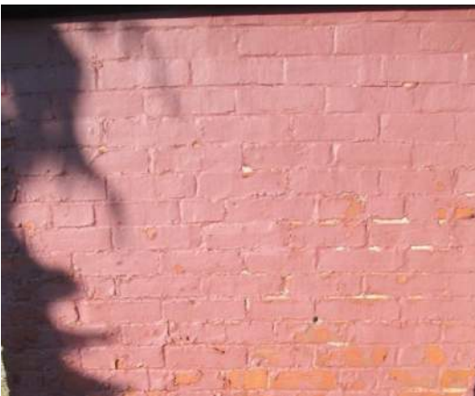
Figure 2 – Above grade brick foundation: far left-hand side (LHS) typical paint failures, peeled and cracked. Plug remains in wall from previous staging support, removal is recommended
