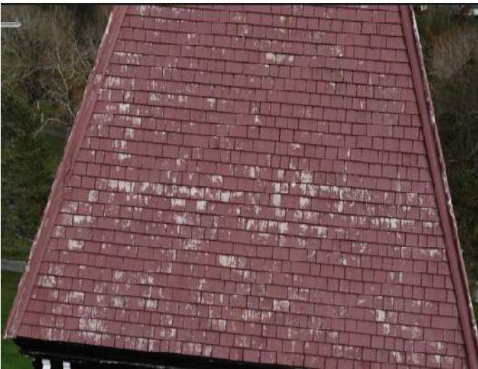
Figure 61 – Tower 1. East elevation. A significant areas of peeled and faded Red Stain
