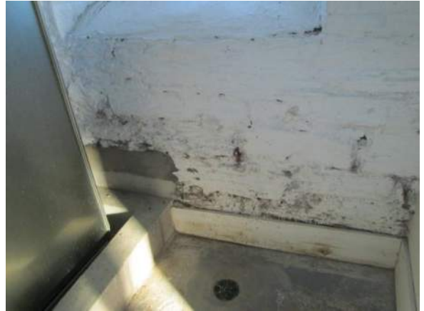
Figure 88 – Oil tank storage room: Newer drain installed to keep water from sitting. Section of wall beyond in wet.
