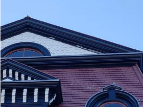
Figure 26 – Paint peeled at gable trim and some locations of stain failures on red roof shingles.
