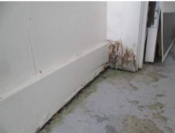
Figure 98 – Wood baseboard is soft and da
