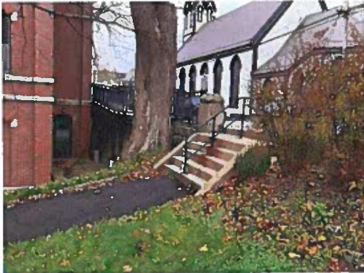
9) Staircase from Townsend Street to the pathway along the east side of Town Hall
