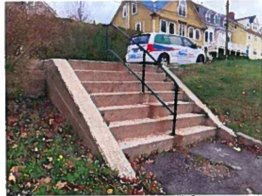
8) Staircase from Townsend Street to the pathway along the east side of Town Hall
