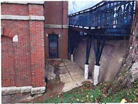
7) Retaining wall and accessible ramp and railing to Town Hall - Townsend Street
