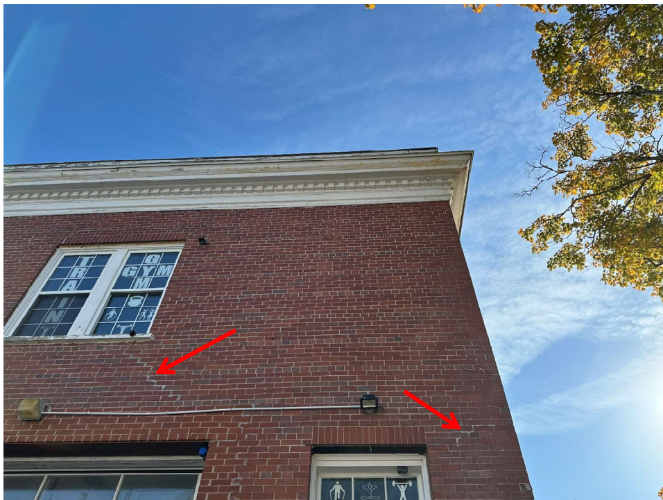
Photo 4: Localized step cracking with touch-up sealant repair attempts
