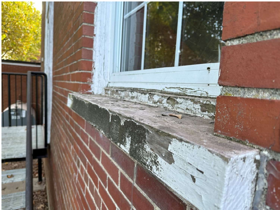
Photo 13: Failing paint finish on exterior window sill (typ. condition at others)
