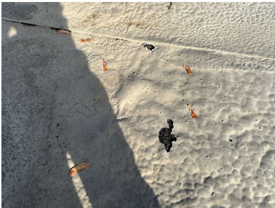
Photo 15: Close up of deteriorated roofing membrane that had a coating applied overtop
