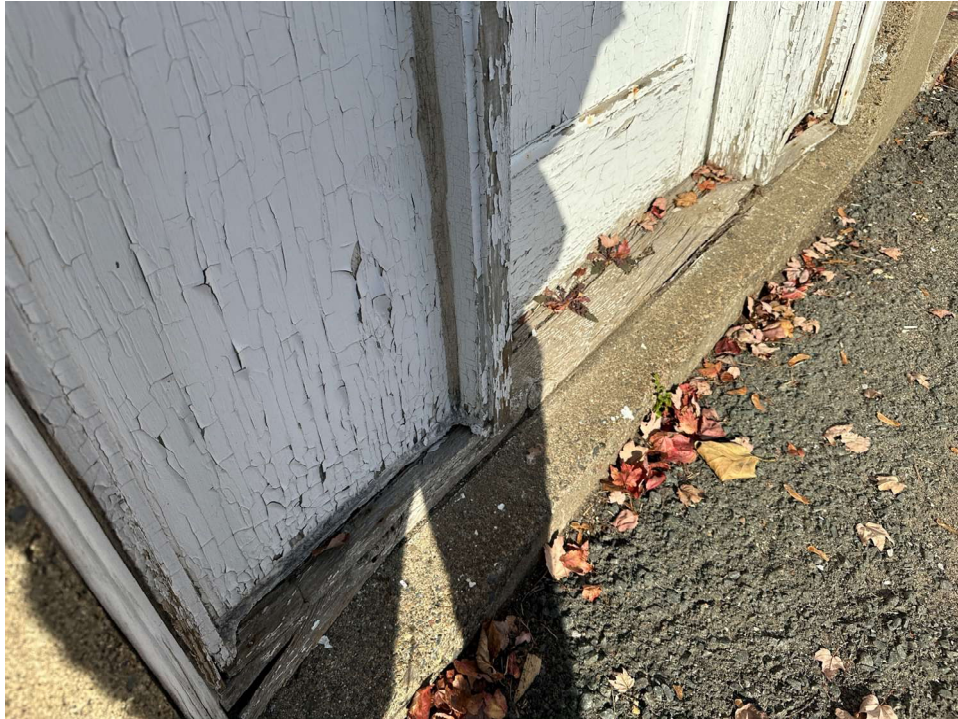
Photo 10: Close up of east elevation door with deteriorated wood threshold and failing paint finish
