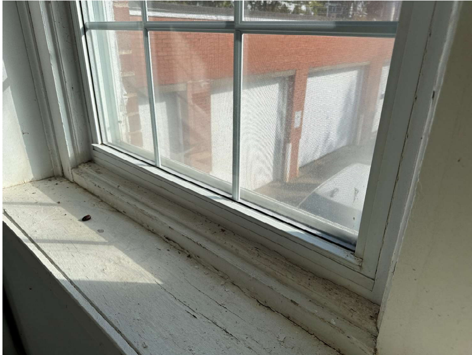
Photo 12: Interior close up of newer vinyl window (typ. throughout building) set in original wood frame in fair to poor condition
