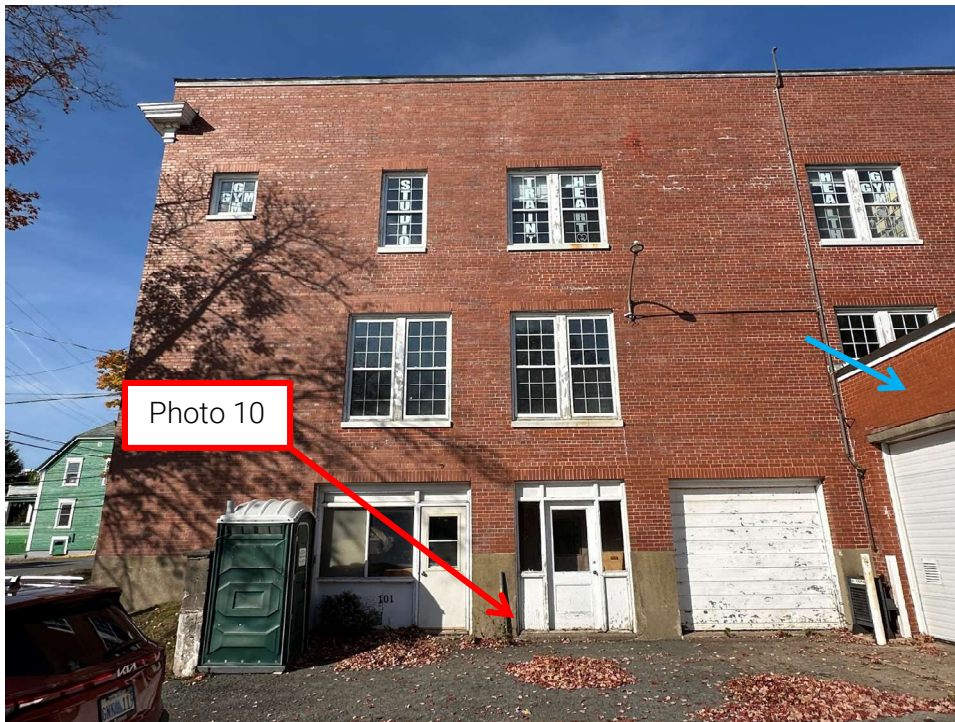
Photo 9: Basement access doors and bay door on east elevation (rear of building). Blue arrow on south wall of Electric Light Shop
