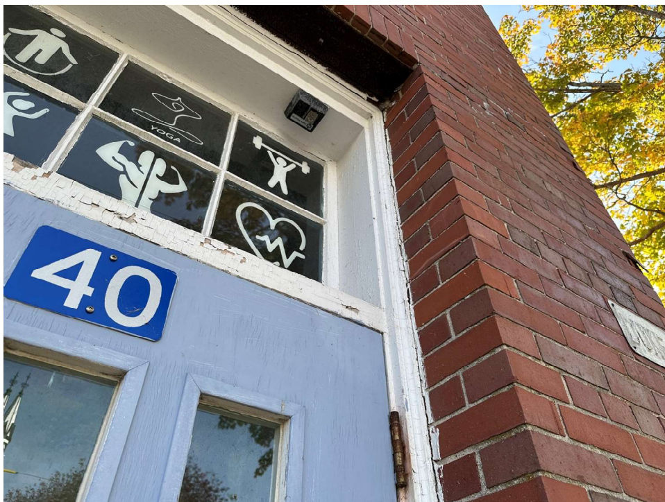
Photo 11: Close up of west elevation door with failing paint finish near southwest corner of building
