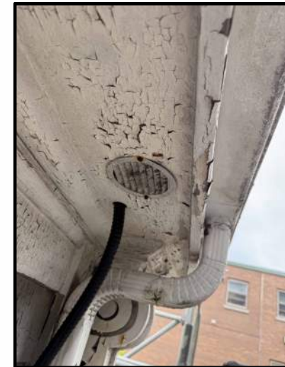
EVIDENCE: ROUND GRILL IN THE LOCATION OF THE DOWNSPOUT THAT WOULD HAVE BEEN CONNECTED TO THE INTEGRAL GUTTER ABOVE.
