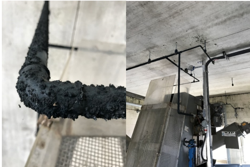
Figure 2 and 3: Existing Water Piping Headworks
