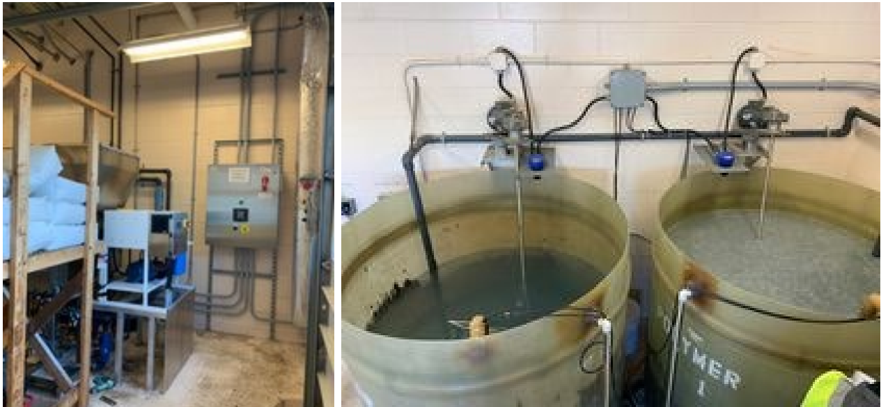
Figure 7 and 8: Existing Polymer Make-down System and Storage Tanks
