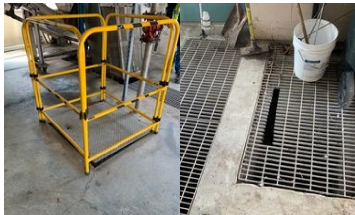
Figure 4: Existing Bilco Hatch to be replaced (left) and example of grating to be replaced (right)
