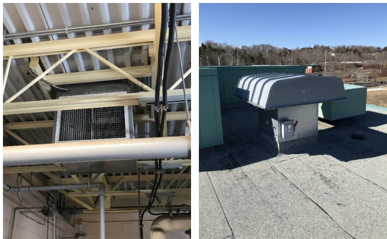
Figure 9 and 10: Existing HVAC equipment to service the blower room
