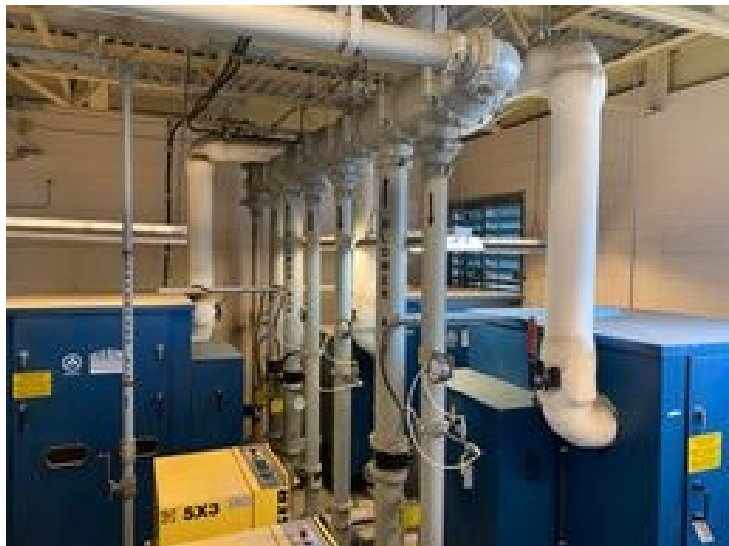
Figure 6: Existing Blower Room
